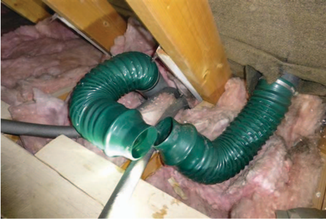
Figure 4: This flexible duct should connect the extract fan from the bathroom to the ventilating tile in the eaves of the roof. Because the wrong ducts have been used, it is impossible to join these effectively allowing warm moist air to get into the roof space
