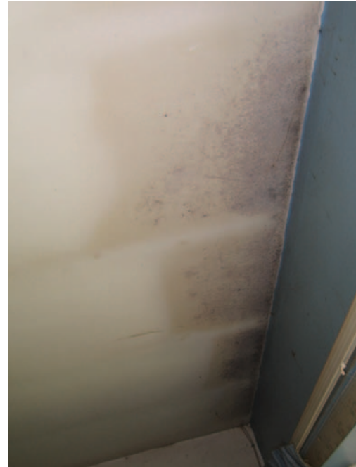
Figure 2: Above this ceiling, the loft insulation has not been pushed up to the back of the wall plate and taken over the head of the wall. Condensation and mould growth has formed on the resulting cold areas. This is still visible despite being cleaned with diluted bleach
