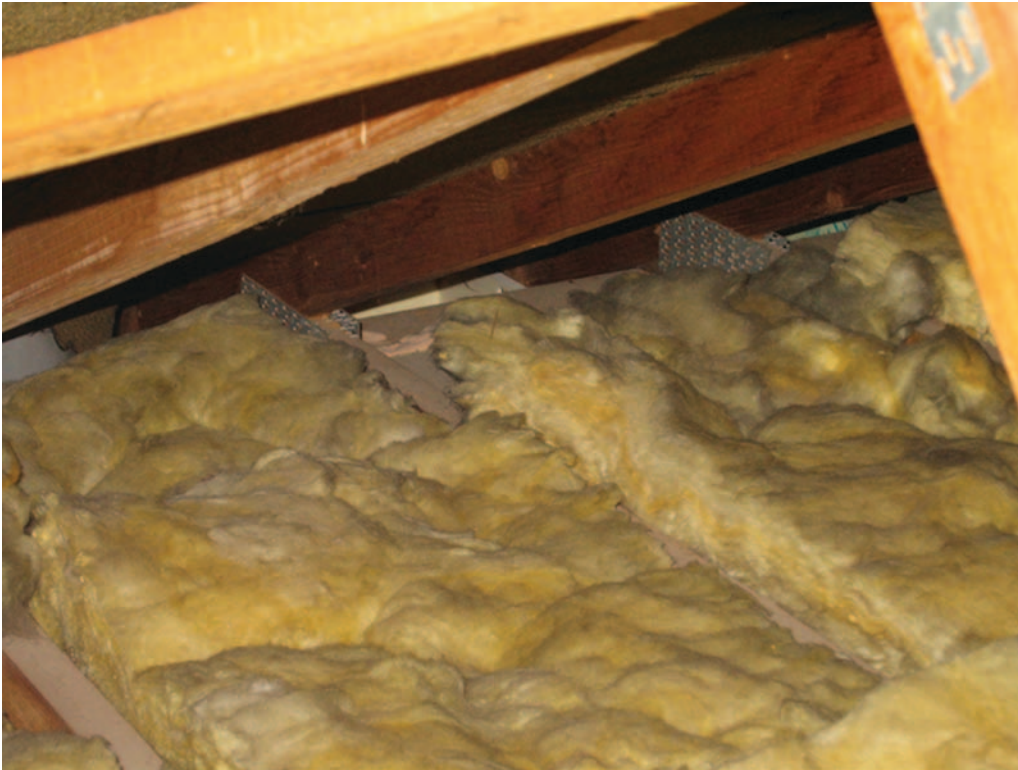
Figure 3: This is the view of the same ceiling shown in Figure 2 but from within the loft space. The insulation is approximately 75mm thick and upgrading this to 250–70mm while maintaining roof space ventilation would be a challenge
